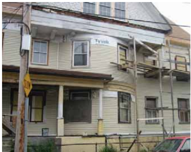
Home in the process of renovation on Hewins Street in Erie-Ellington area of Dorchester.
