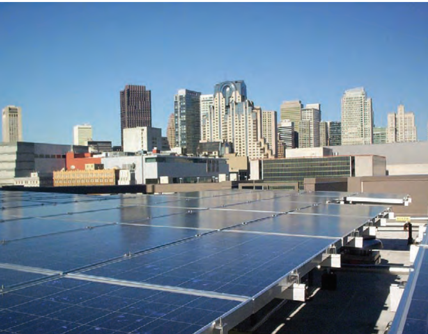
Plaza Apartments in San Francisco. A view of the rooftop solar panels on this mixed-use development that includes low-income housing.
